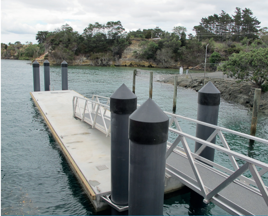
Kennedy Point Marina Attenuator Piles installed by Heron Construction Co. Ltd, New Zealand
